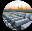
Power & Data Infrastructure
